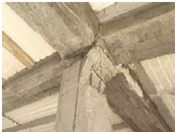
Figure 2. Spalling of column concrete and undamaged beams (Vetr et al., 2018).
