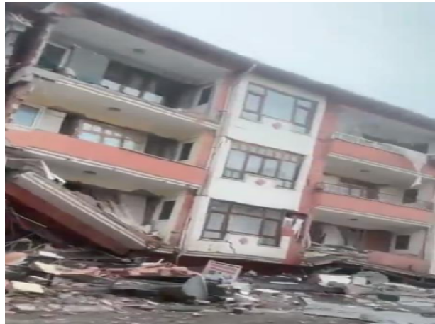
Figure 1. Collapse of a residential building due to column failure (Sezen et al., 2023).
