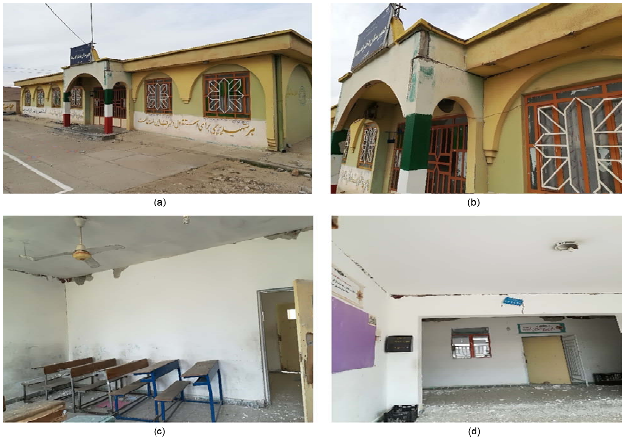
Figure 8. A case of detachment between roof and supporting wall led to a reduction in the seismic forces acting on the masonry walls.
