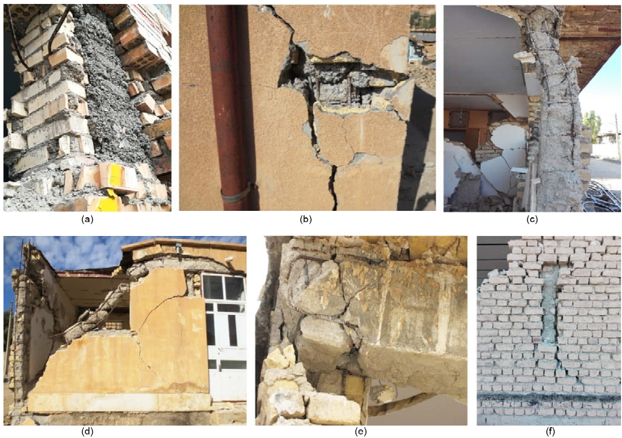
Figure 9. Instances of defects in confining elements and resulting damages.
