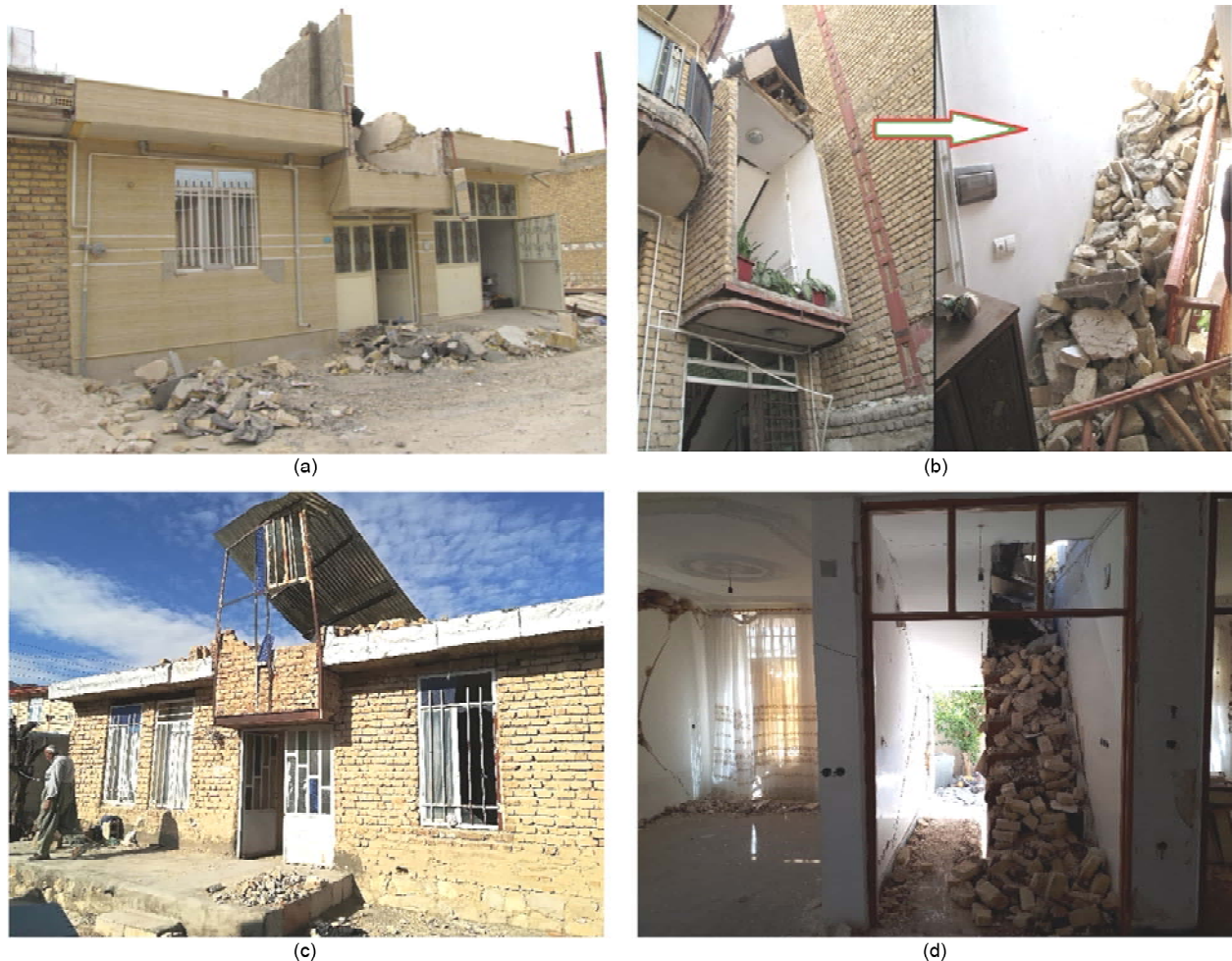
Figure 14. Instances of failures in roof access enclosures.
