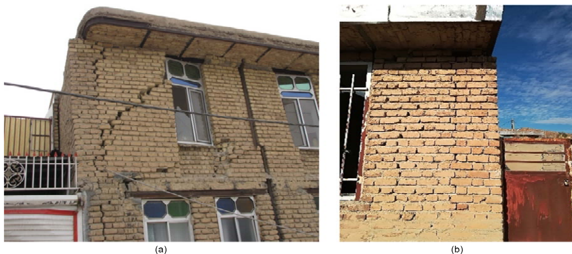
Figure 7. Disconnection between roof and supporting wall.
