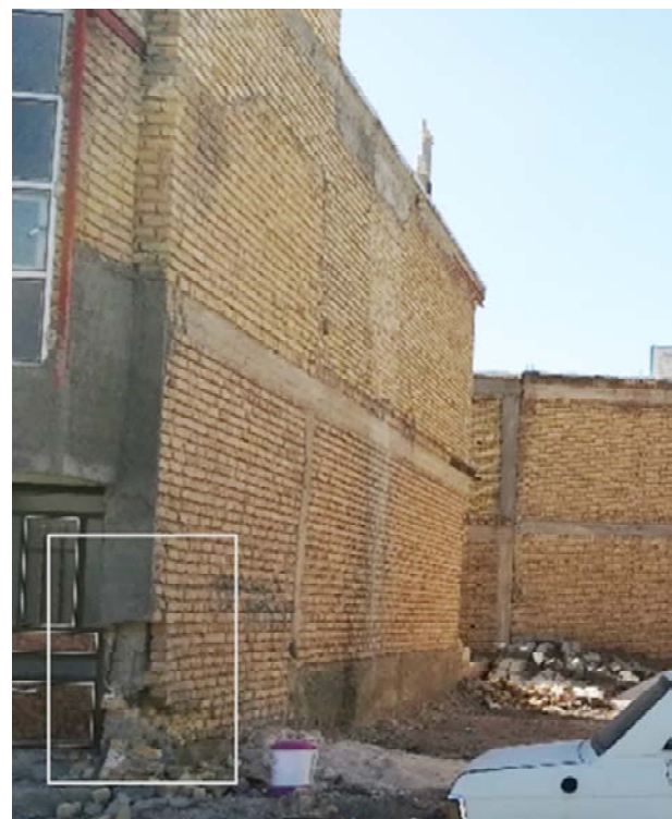
Figure 21. Instance of flexure failure mode in CM wall.
