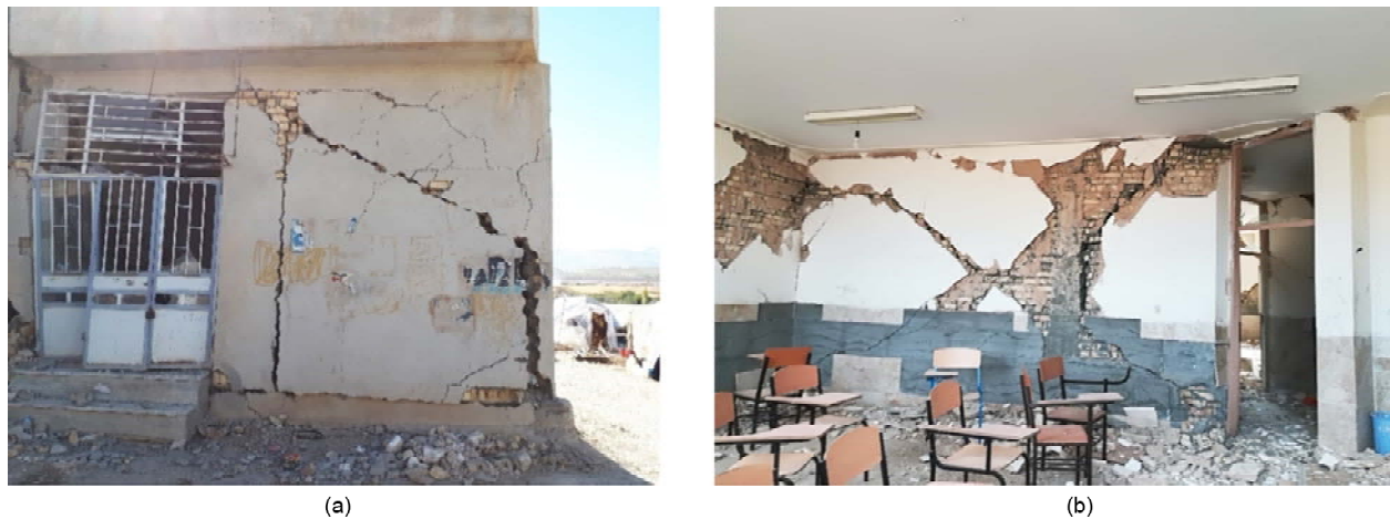
Figure 20. Instances of shear failure of confined masonry walls.
