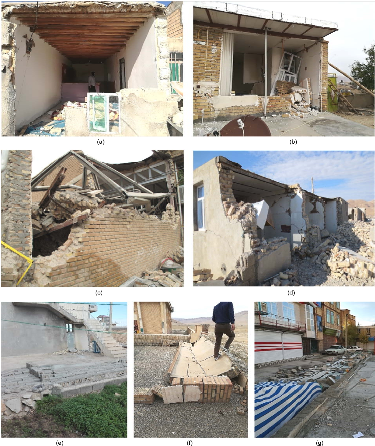
Figure 13. Instances of OP failure of URM walls.
