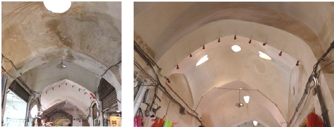
Figure 5. The permeation of moisture on the arches, vaults and domes.
