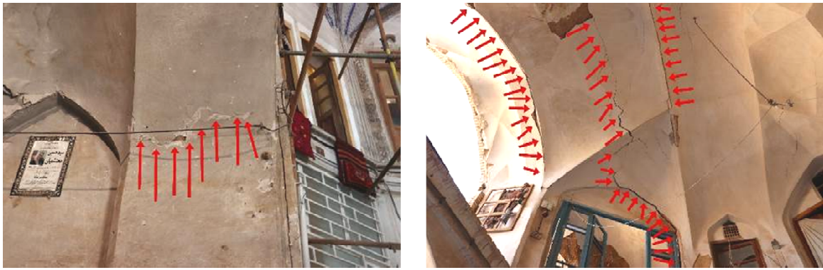
Figure 4. Deep cracks in the arches and vaults.
