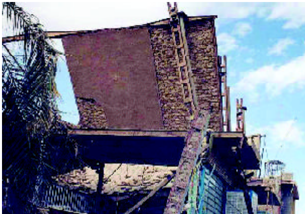
Figure 10. Integrity of the anchored jack arch slab under earthquake loading and after collapse.
