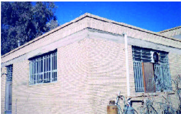
Figure 14. No damage in this code-designed masonry building having ring-beam supported, jack arch slab.
