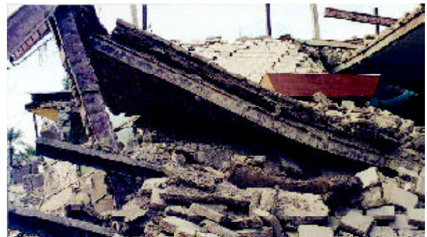
Figure 12. Ability of the anchored jack arch slab to undergo large deformations.
