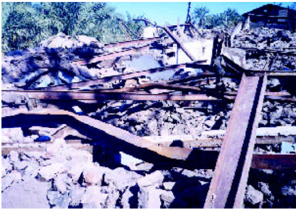
Figure 7. Collapse and disintegration of unanchored jack arch slabs.
