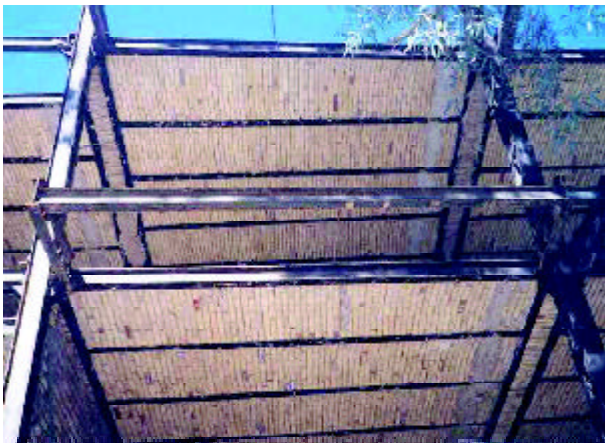
Figure 15. Good seismic performance of anchored jack arch slabs made with lightweight perforated bricks.
