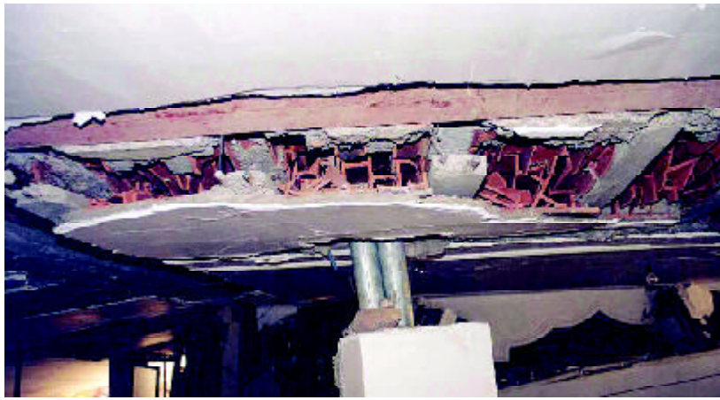
Figure 18. Lack of proper connection between the slab concrete beams and the steel support beam.
