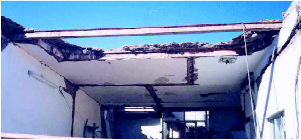
Figure 16. Effectiveness of inter-span transverse beams in keeping the integrity of the slab.
