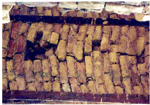
Figure 9. Failure of masonry arch as a result of out-of-plane bending loads.
