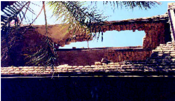
Figure 8. Failure of masonry arch due to in-plane transverse loading.
