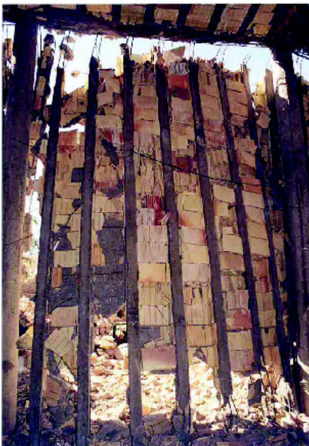
Figure 19. Poor workmanship in construction of concrete beam-hollow block slab.
