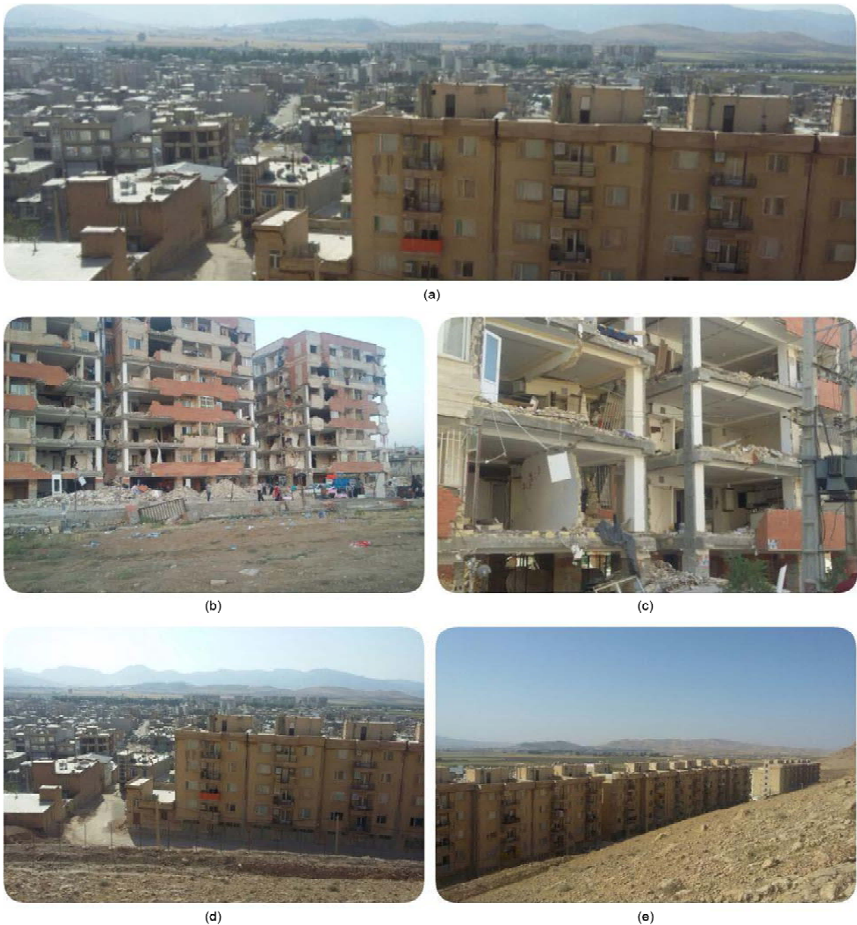
Figure 2. West of Sarpol-e Zahab city, (a) structural damages most likely to be affected by the local site effects, (b, c) buildings near to the river, (d, e) buildings near to the mountain.
