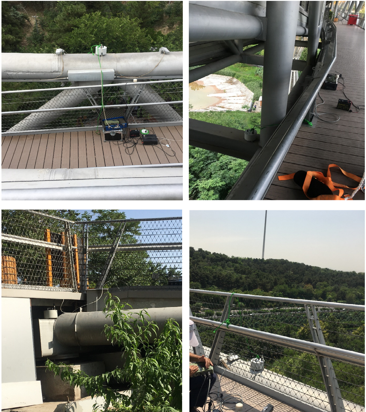
Figure 3. Seismic sensor along with the data logger and other accessories.
