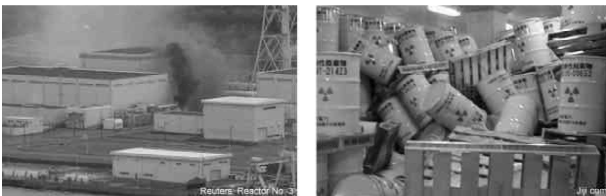
Figure 18. Fire in an electrical transformer at the nuclear power plant and displaced barrel of nuclear waste. The radioactive materials were also leaked to the ocean and contaminated the environment.
