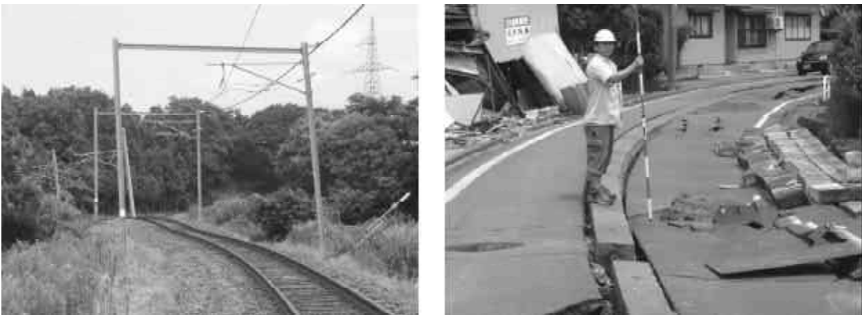
Figure 11. Settlement of the railway embankment in Doh-Ai and damaged road pavements near the railway.
