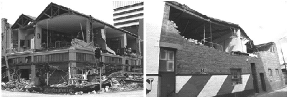
Figure 4. Typical out of plane failure of solid masonry walls in the September 2010 earthquake.
