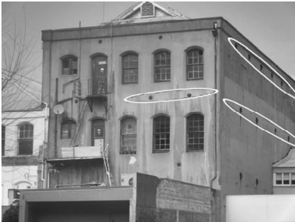
Figure 9. URM building with walls anchored to the floor/roof via a grid of bolted anchor ties.
