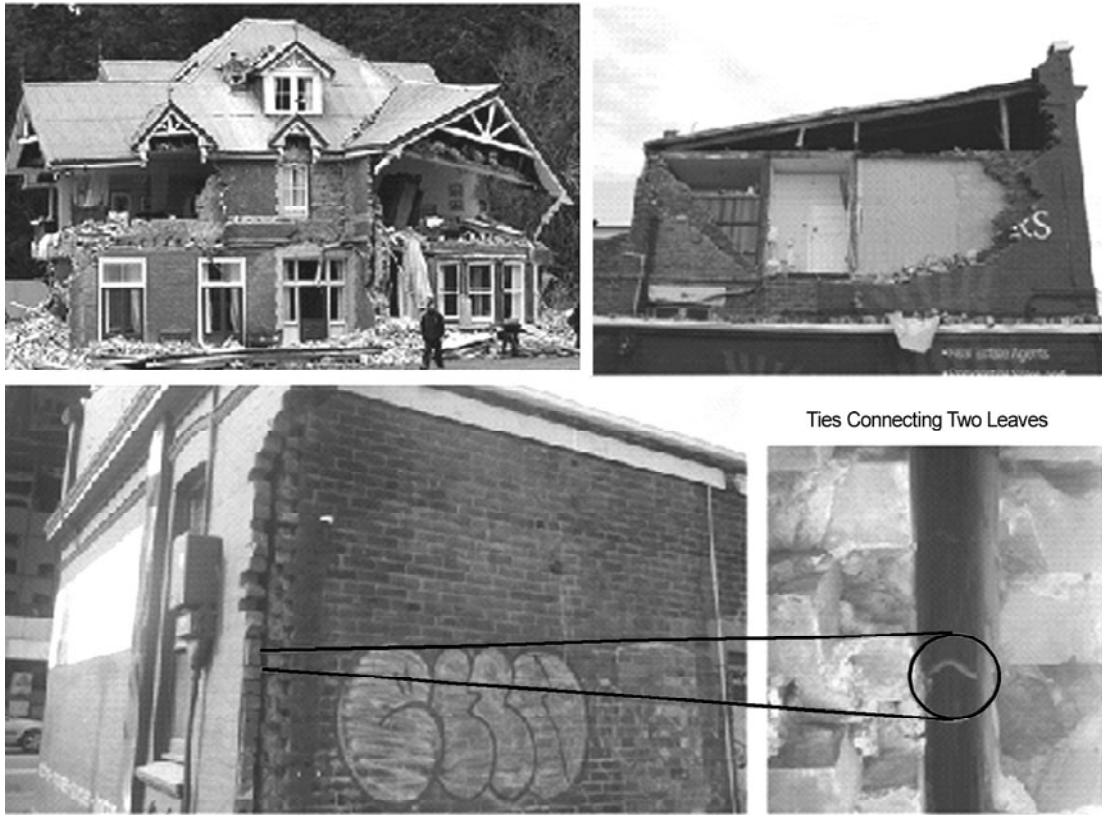
Figure 5. Typical failure of cavity walls in the September 2010 earthquake.
