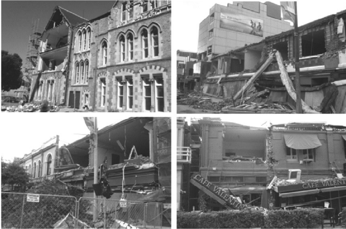
Figure 15. Out-of-plane failure of URM walls observed in the February 2011 earthquake.
