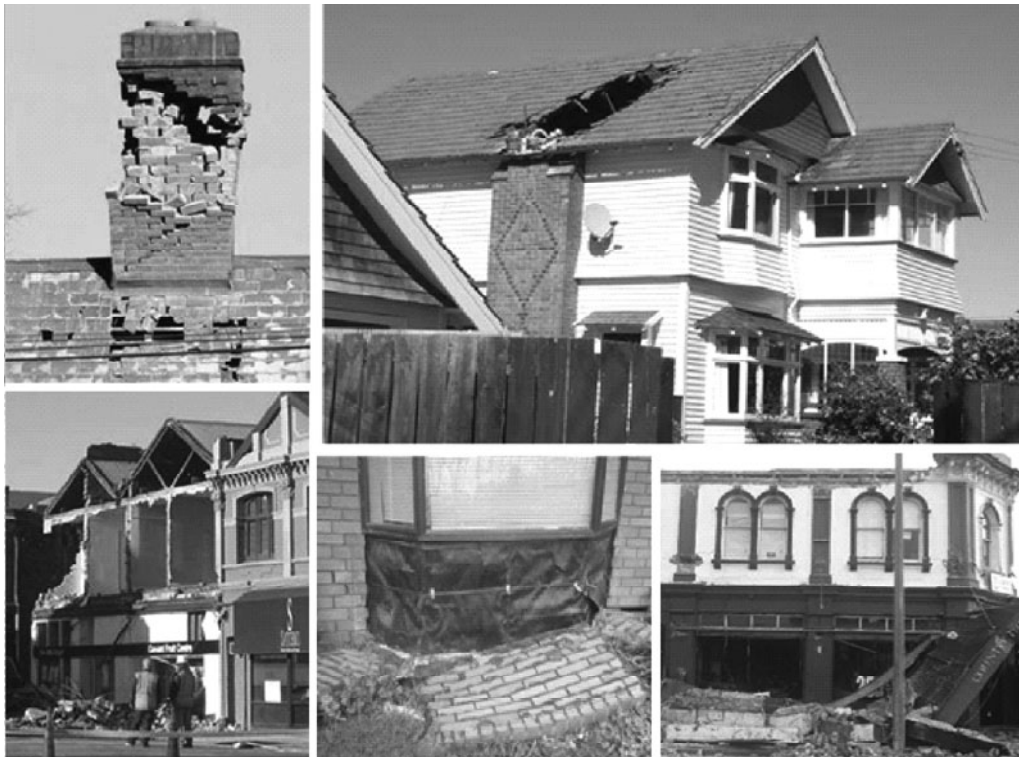
Figure 8. Failure of brick masonry chimneys, facades, walls and parapets observed in the September 2010 earthquake.
