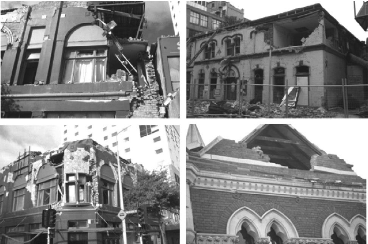
Figure 21. Performance of inadequately anchored masonry walls in the February 2011 earthquake.
