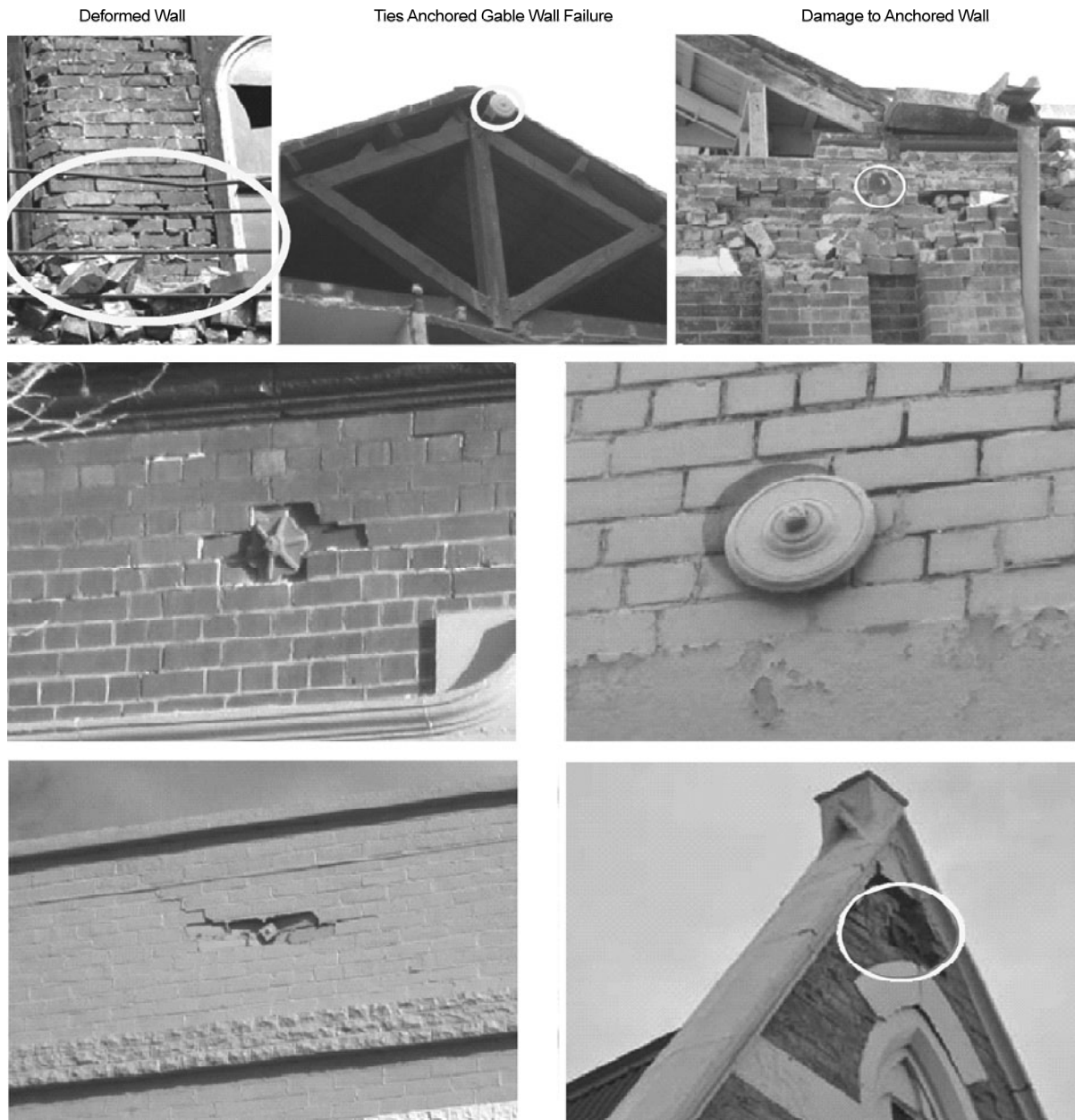
Figure 13. Typical damage to anchored walls observed in the September 2010 earthquake.
