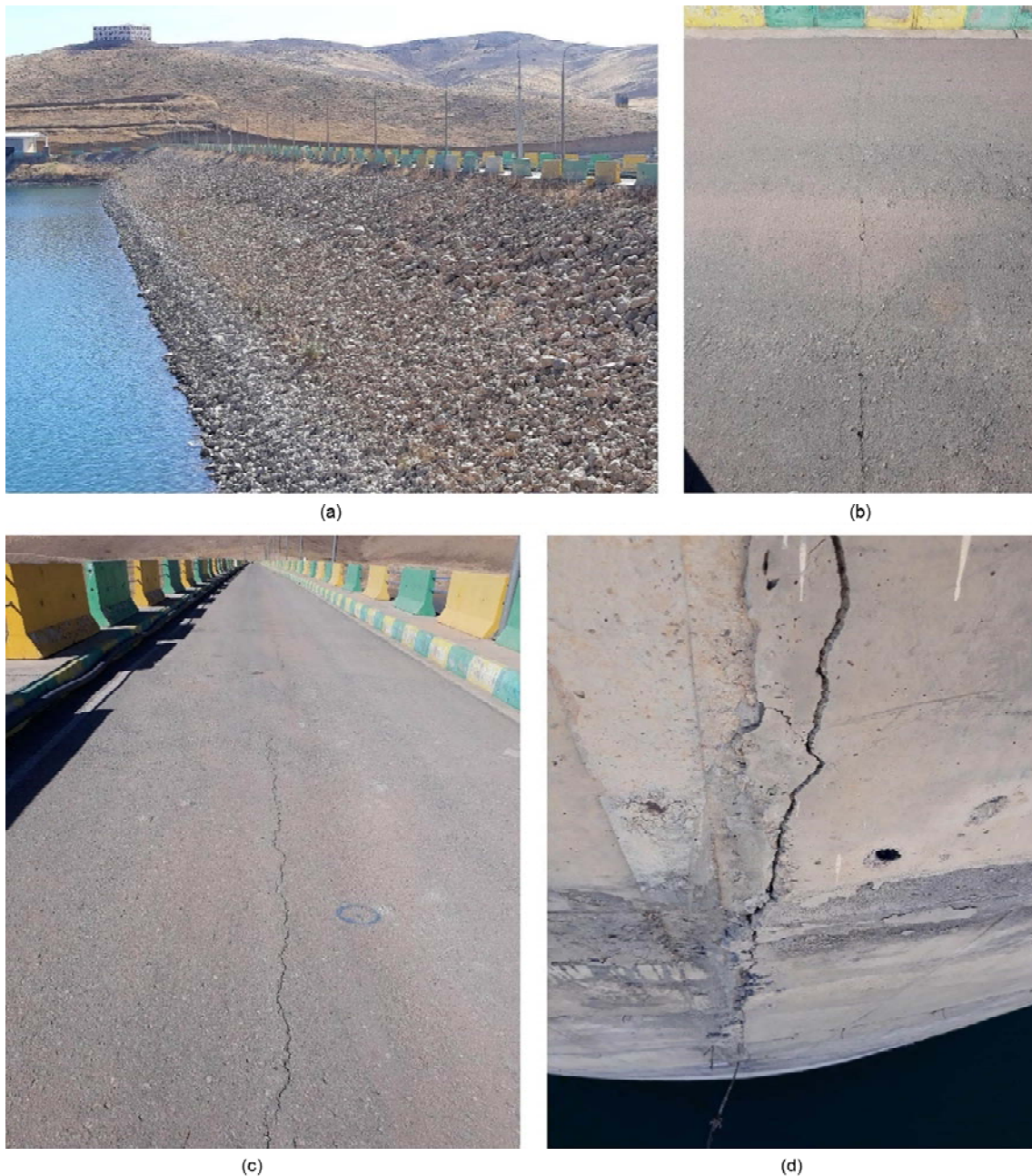
Figure 4. Images of observed cracks in Tange-Hamam Dam, (a) General view of the dam after the earthquake, (b) very small tiny transversal crack on the crest, (c) Longitudinal Crack on the crest, and (d) Crack and separation on the concrete at a joint place of the left wall of the spillway.
