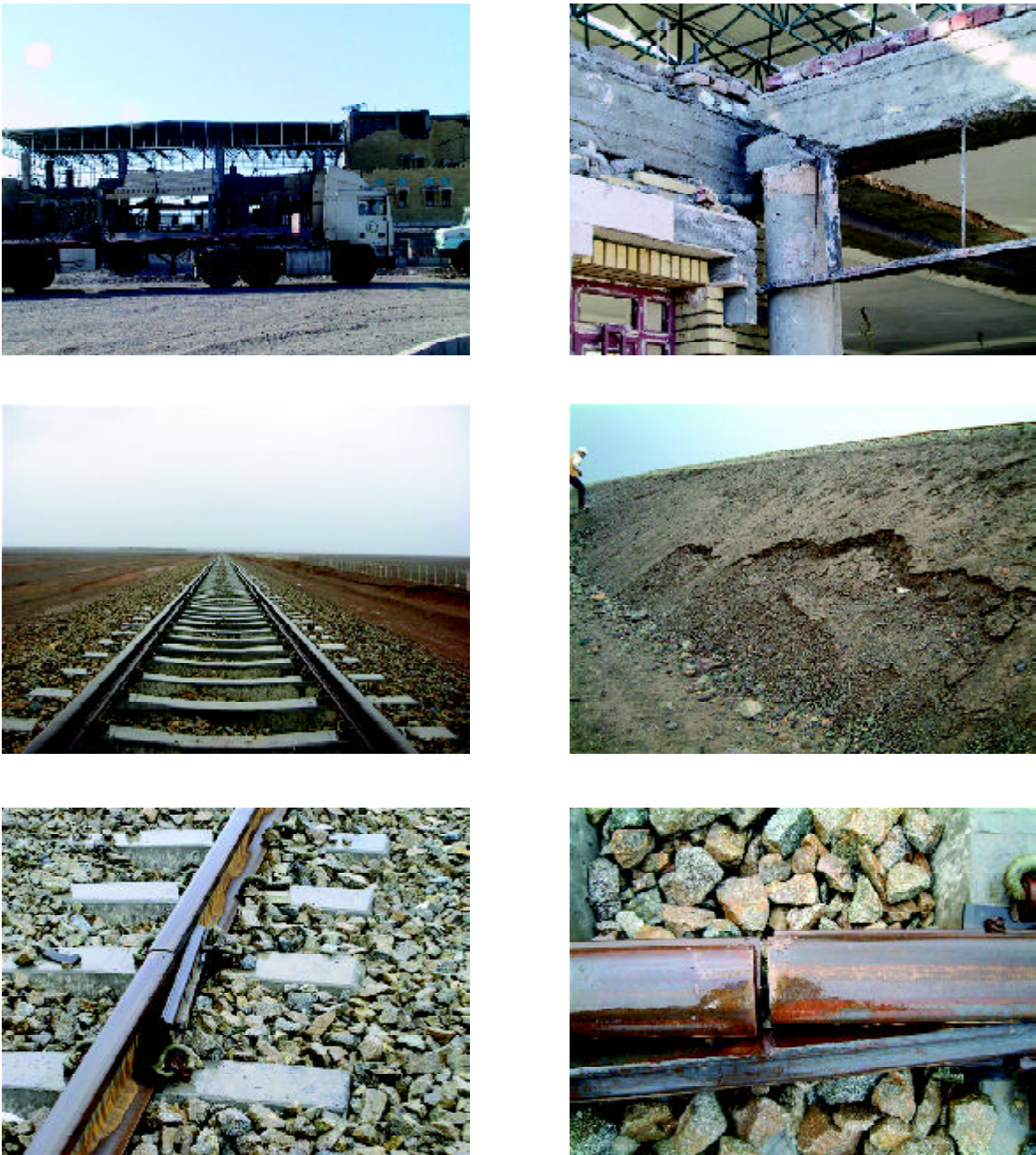
Figure 13. The passenger terminal was under construction and had minor damage. There was no damage to rail tracks. There was light damage to embankment.
