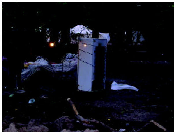
Figure 9. Damage to various electric equipments in the 230kV substation is observed in the above pictures. At the time of our visit (one month after earthquake) the electricity was available throughout the city, even though most of the users' buildings had been severely damaged to use the electricity.
