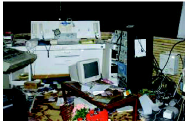
Figure 45. The failure of mechanical and electrical facilities and interior equipment of the Bam airport control tower (Photo Source: http://www.irna.ir/melli/bam/photo_index6.htm )
