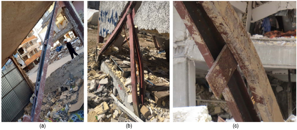
Figure 5. Lack of connector plates or brace-to-connection plate welding in brace members with double channel section.
