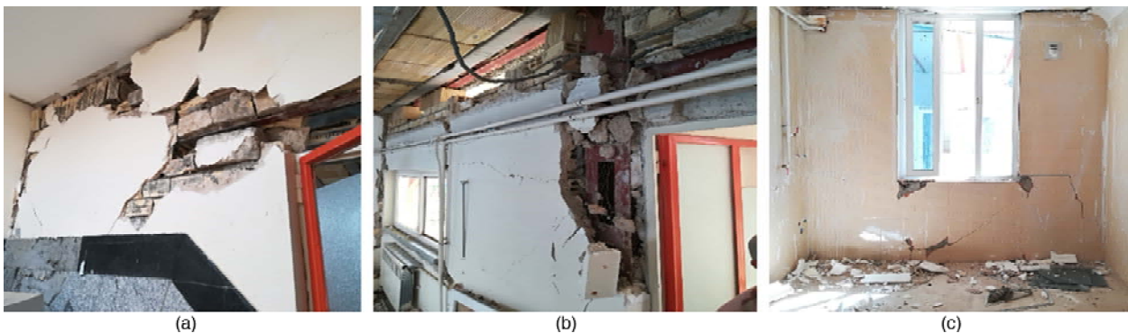
Figure 22. In-plane failure of infill walls.
