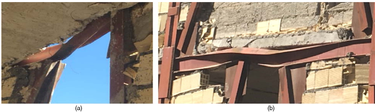
Figure 18. Lateral-torsional buckling of link member due to the lack of lateral bracing of link member.
