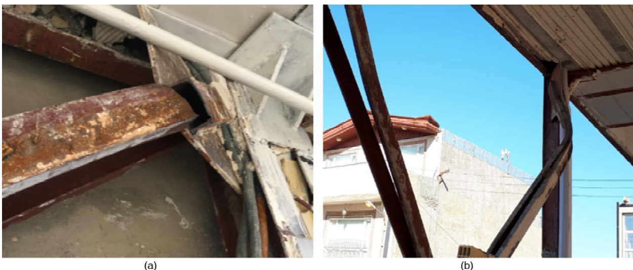
Figure 4. Premature buckling of brace members due to the excessive out-of-plane deformation in gusset plates.
