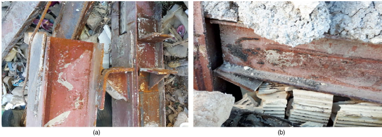
Figure 15. Common Brittle failure modes in moment connections. (a) Weld failure at the flange plate-to-column. (b) Weld failure at the flange plate-to-beam.
