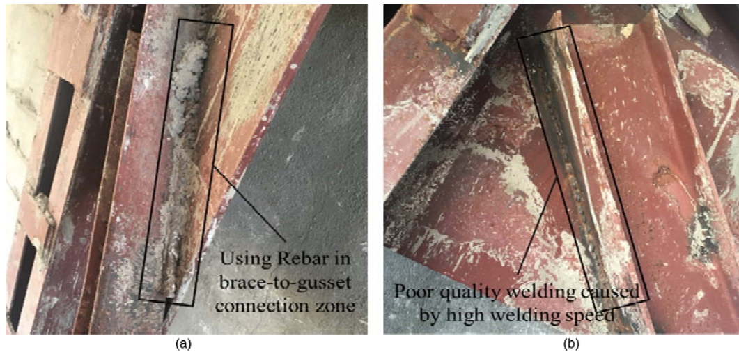
Figure 11. Poor quality of welding in brace connections.
