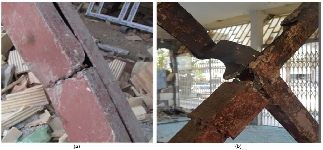
Figure 7. Inappropriate brace splices.
