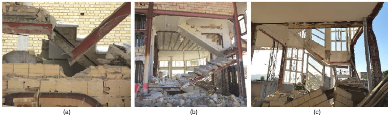
Figure 24. Failure of staircase.
