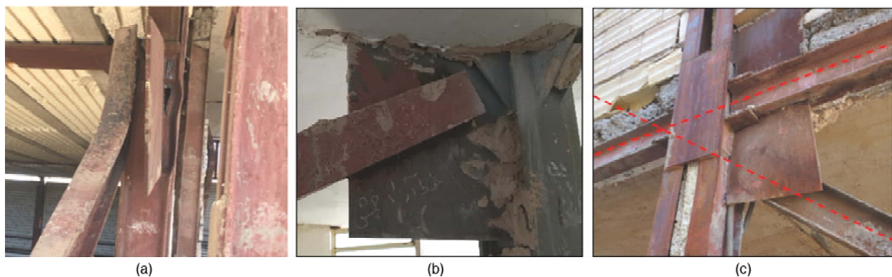
Figure 12. Inappropriate geometrical detailing of gusset plate. (a) Out-of-plane eccentricity in the brace connection. (b) Ignoring fold line in gusset plate, necessary to accommodate significant rotations corresponding to out-of-plane buckling of brace. (c) In-plane eccentricity of brace to beam-column joint.
