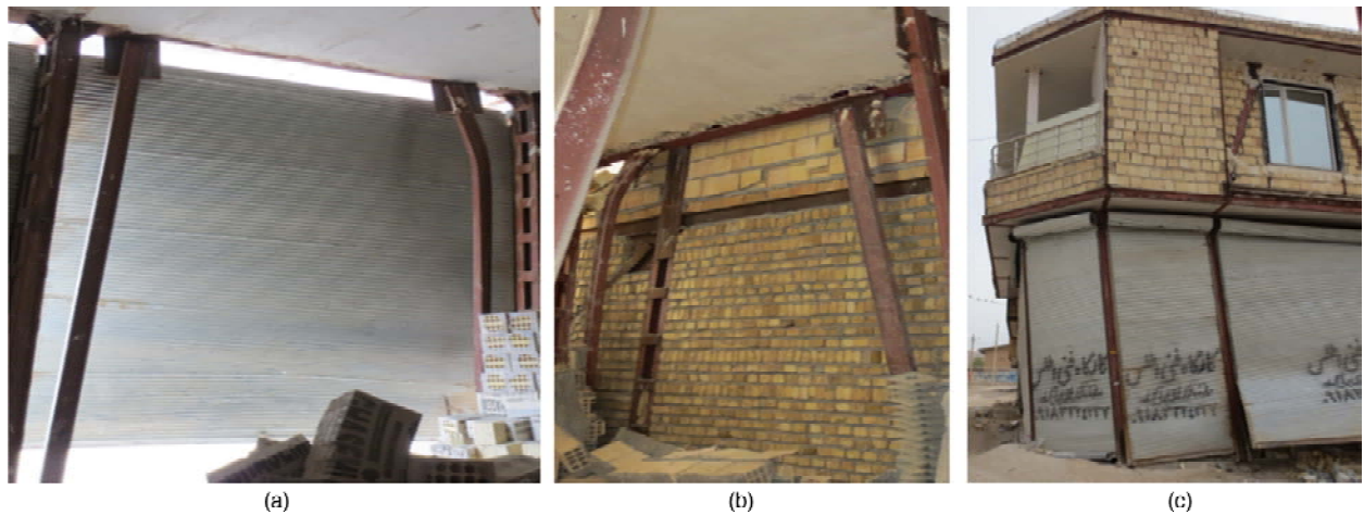
Figure 20. Case study: A 2-story eccentrically braced frame building with excessive eccentricity ratio.
