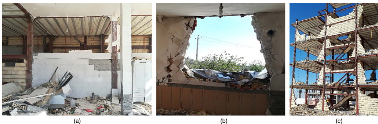
Figure 23. Out-of-plane failure of infill walls.
